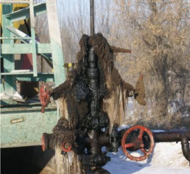
Water and oil leakage
